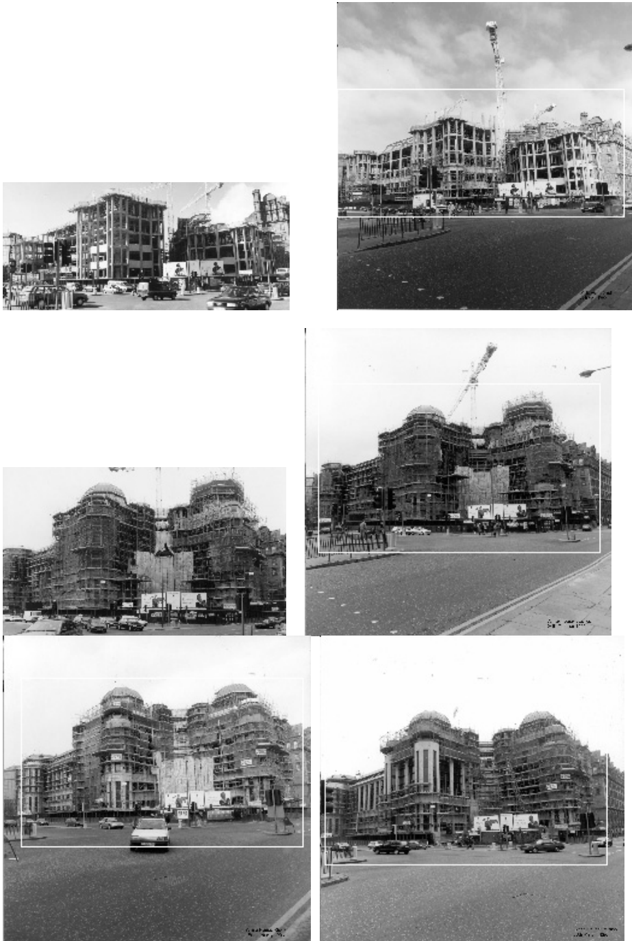
Figure 7. Top left: model of the building in progress, March 1995. Top right: located model in same-viewpoint photograph taken in April 1995. Middle right: model of the building in progress, September 1995. Middle left: located model in same-viewpoint photograph taken in October 1995. Bottom: September model located in January and March 1996 photographs
