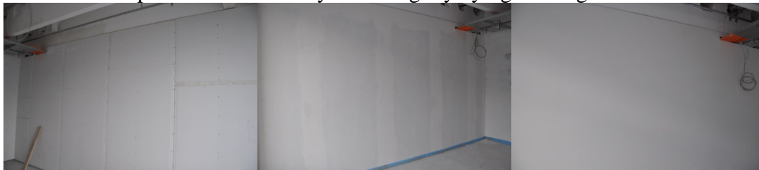
a) b) c) Figure 1. Example image of a) installed drywall panels, b) plastered drywall and c) painted drywall
