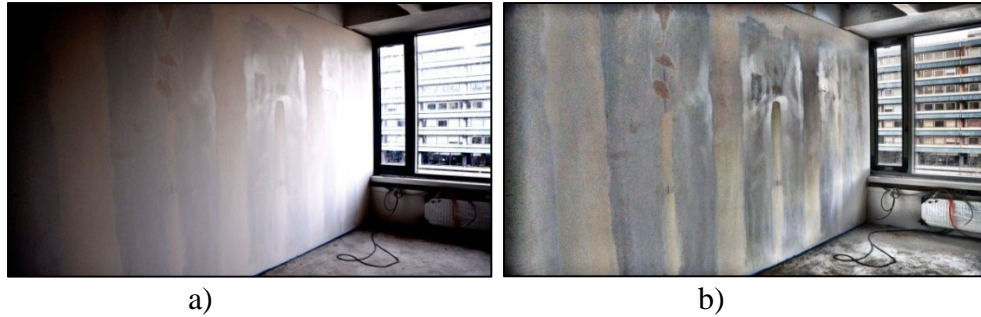
Figure 6. Example of a) original plastered drywall image and b) adaptive histogram equalized image
