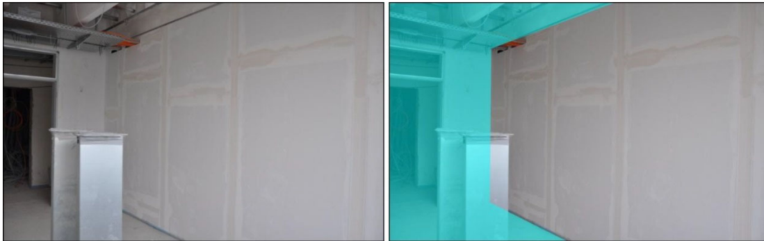
Figure 2. Example image of a drywall with original appearance (left) and BIM extracted ROI (right).
