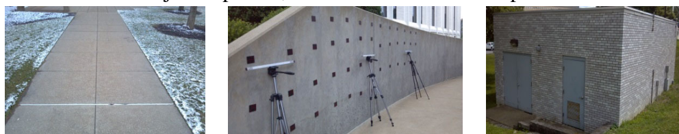
Figure 2. Left to right: a) Sidewalk slab, b) Retaining wall, c) Storage building
