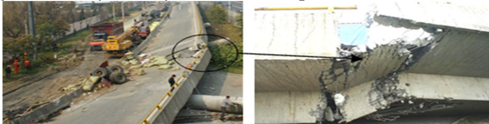
Figure 4. The failure pattern of box girder at collapse scene
