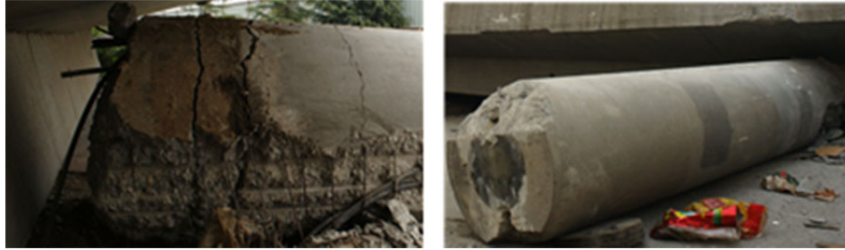
Figure 2 Failure pattern of pier at collapse scene
