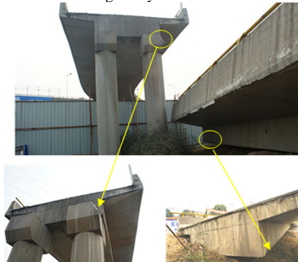
Figure 7. Wreckage collision traces of box girder at collapse scene
