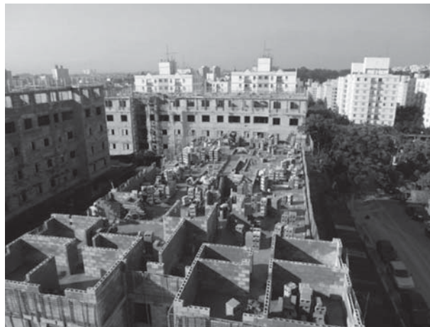
Fig. 2.2 Image from the construction work in which the case study was developed
